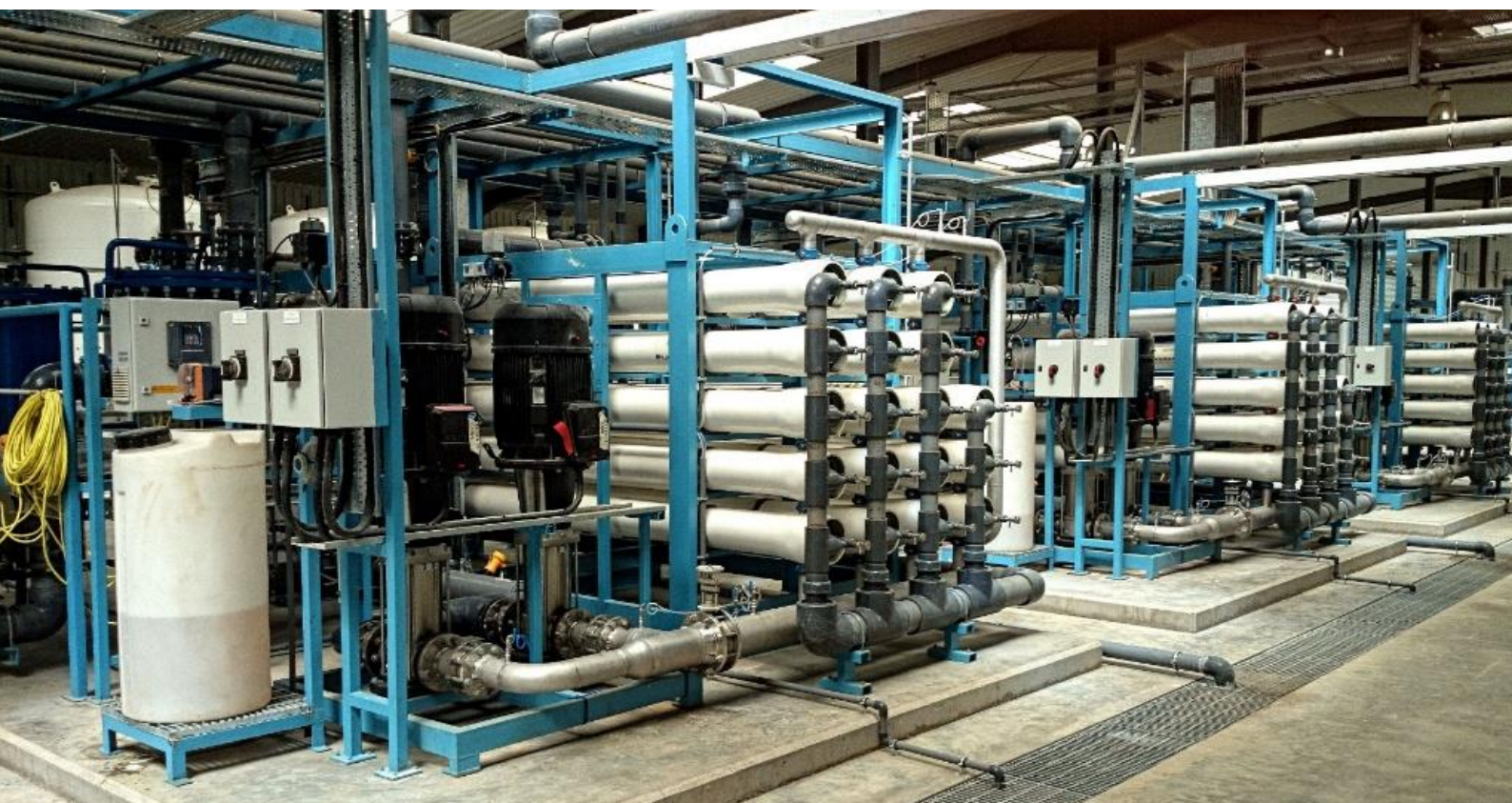
Reverse Osmosis Desalination Plant
